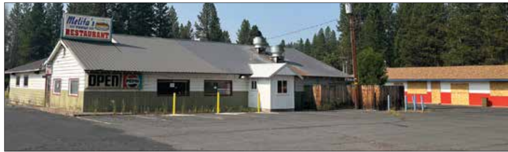
Work will begin to renovate the former Melita's Restaurant where The Klamath Tribes are going to operate a restaurant for food distribution and warm meals for elders, and a community gathering place. (Ken Smith/Klamath Tribes News)
