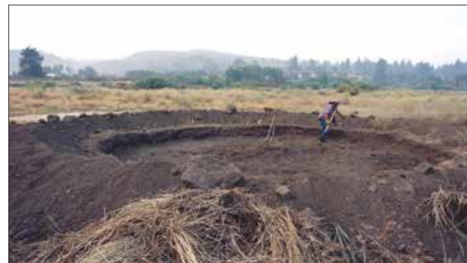
Ivan Jackson digging the footprint of the earth lodge by hand. He dug it to about 40 feet or so wide by 4 feet deep. When finished it required a ladder to get into and out of, and was about twice as tall as Ivan's head above the center pole. (Photo courtesy of Mary Williams Hyde)
