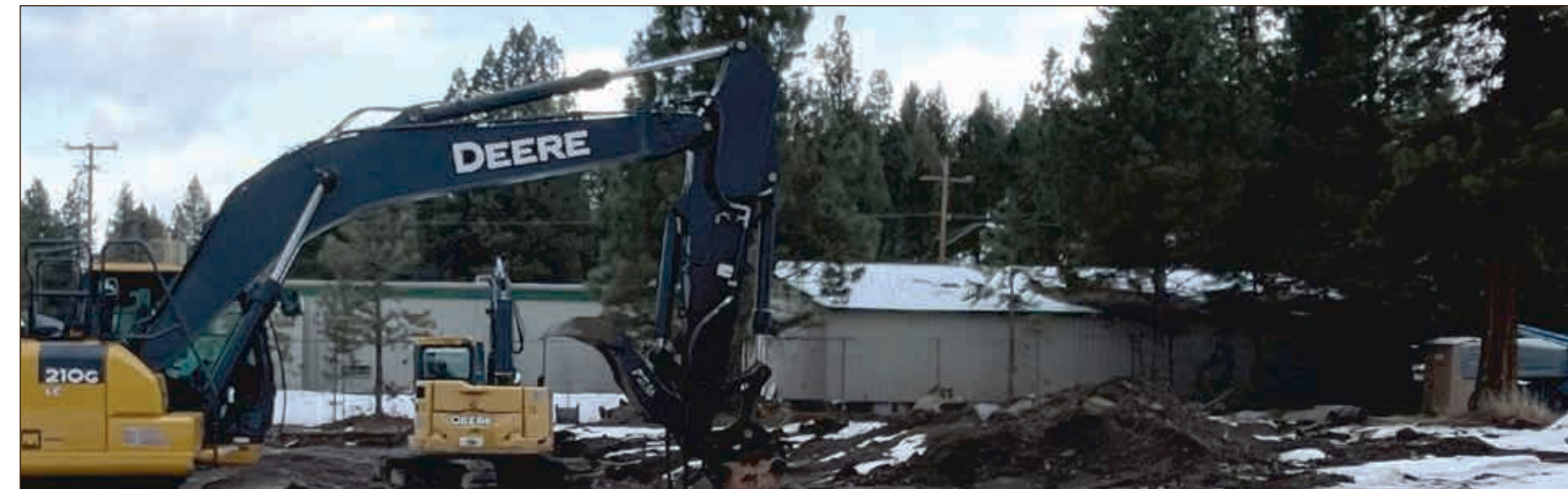
Construction is underway downtown Chiloquin. The triplex will provide three homes for tribal elders, will be downtown between Chocktoot and Yahooskin Streets, while the fourplex, providing another four families with homes, will be situated on Juda Jim Street. (Ken Smith/Klamath Tribes News)
