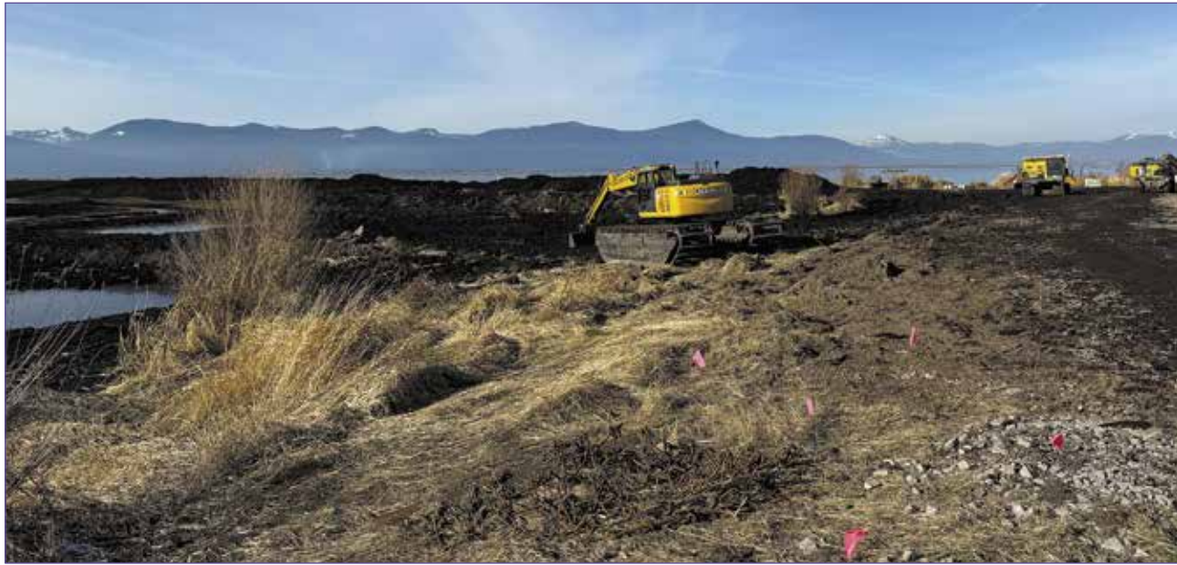
Excavation work is ongoing at the Agency-Barnes site where several breaks in the levy are allowing water to flow from Agency Lake into Upper Klamath Lake, and creating new marshlands. The project is expected to be completed in December 2025. (Ken Smith/Klamath Tribes News)
